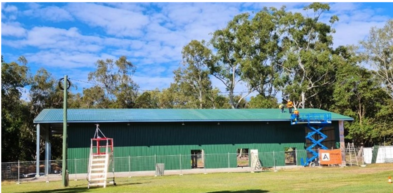
Figure: The Lava Blue research facility under construction in Redlands, Brisbane. The 440 sq m, 6 m high, steel structure will be operating early in 2022 and will conduct repetitive process validation operations, producing 20kg batches of HPA from various materials while developing process control options for commercial scale production.
