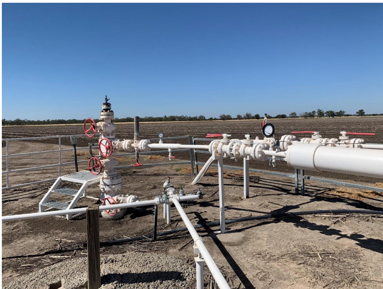
Figure 3 - Myall Creek well head and surface infrastructure
