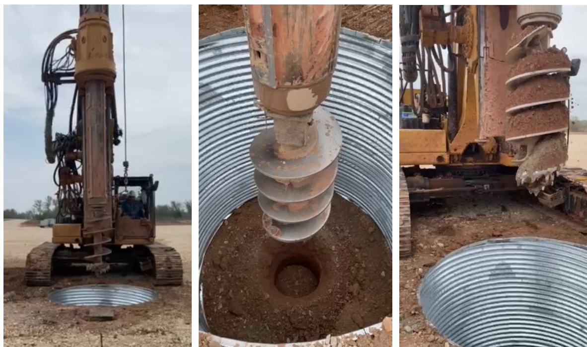
Figure 1. Drilling of the Jewell Well conductor casing hole using a specialised auger drill
