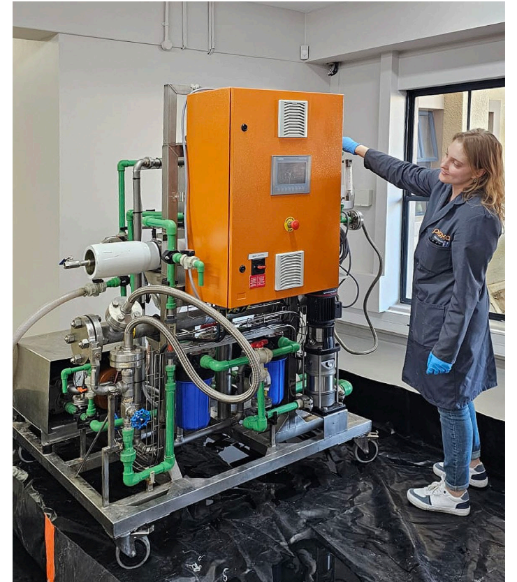
Waste-Water equipment trials, PSG Demonstration Facility
