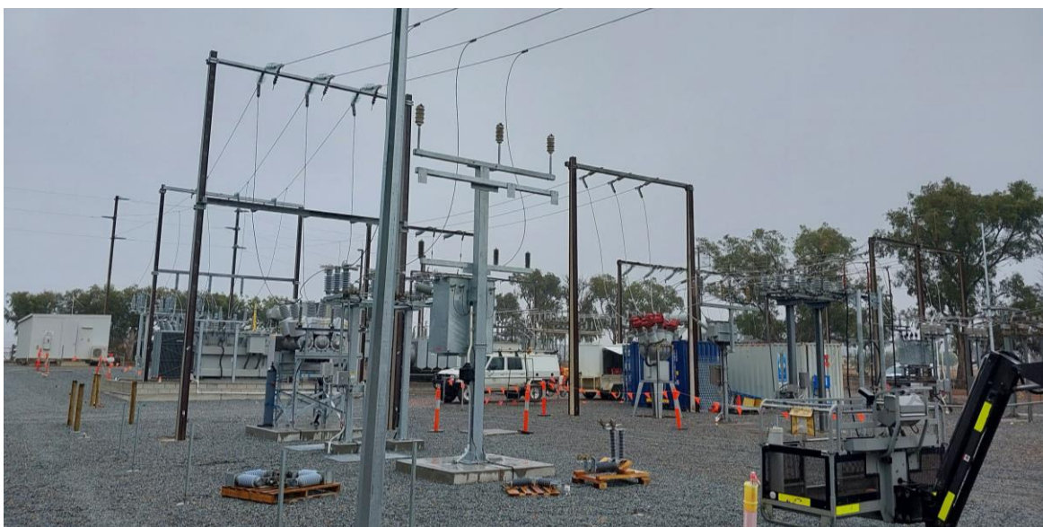
Figure 1. Upgraded Cleve Substation
